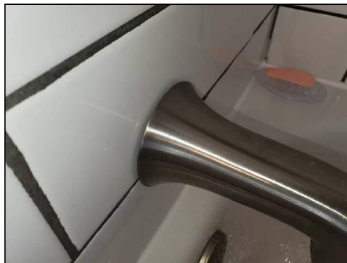
2. Caulking loose, missing or deteriorated
