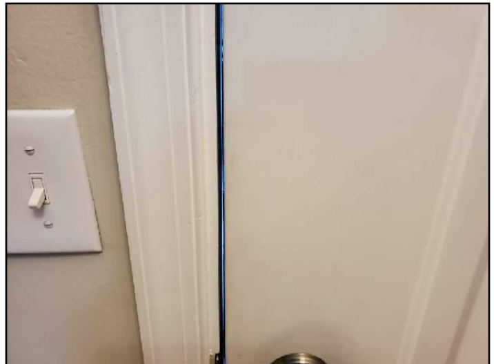
5. Weatherstripping missing or ineffective
