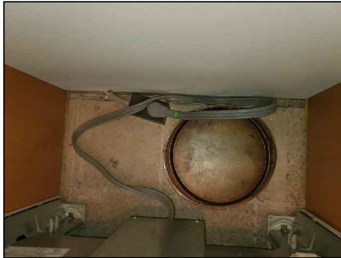
9. Anti-tip device missing
