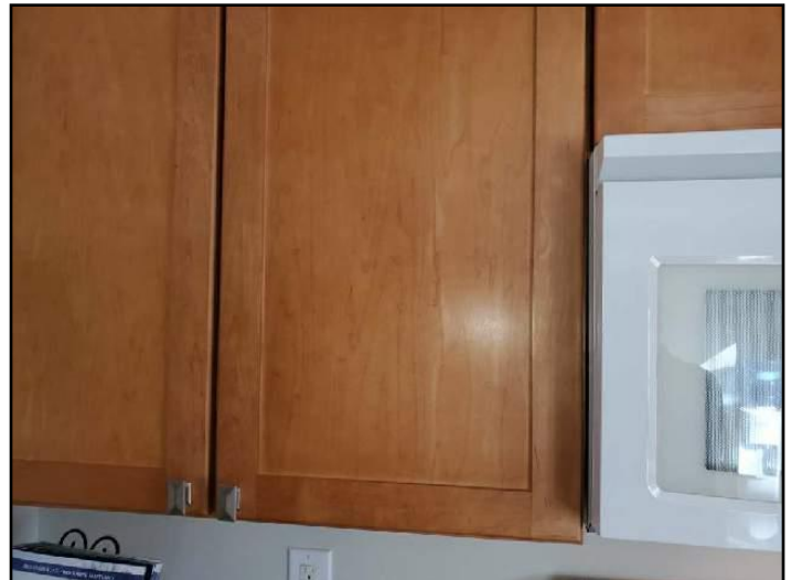
8. Doors or drawers missing or loose
