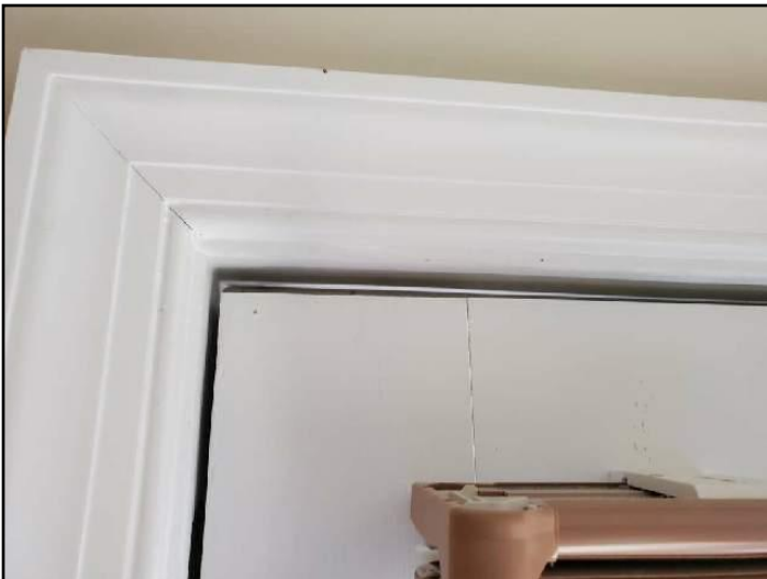
4. Weatherstripping missing or ineffective
