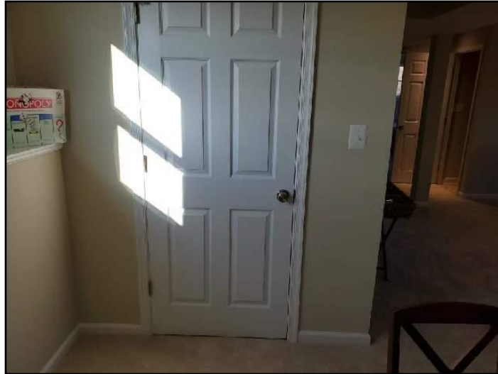
6. Does not latch properly
